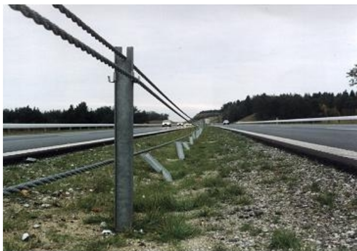
Wire Rope Safety Fence: here, one of the cables is not in place, following an accident
