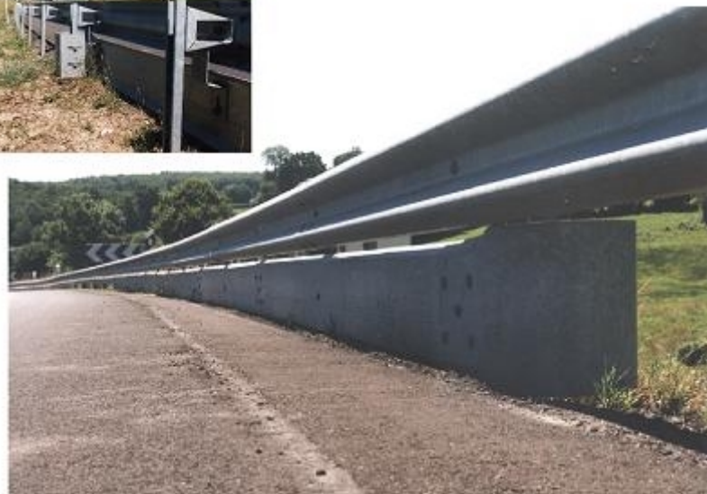
On a French road, a second lower flat rail is fitted under the armco (above: rail seen from behind)
